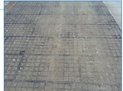
5 Topsoil is added to the open cells and brushed so the top of the cells are not covered by soil. This will allow the cell walls to protect the vegetation from the weight of the fire truck.
