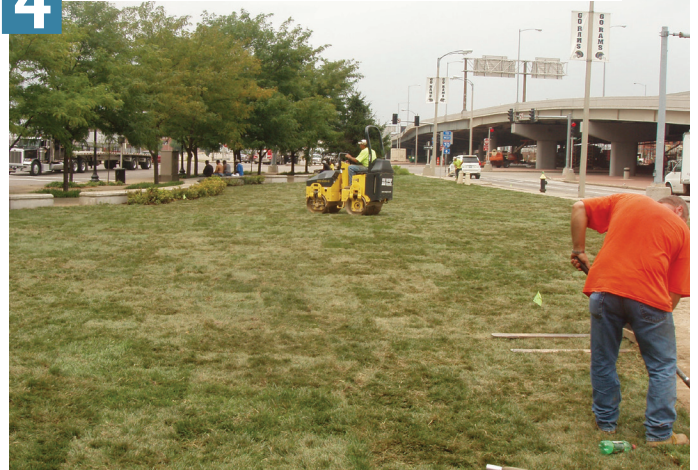
4 Sod was placed on top of the soil filled cells and rolled.
