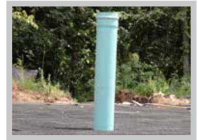
Fig. 12 Installed maintenance port
