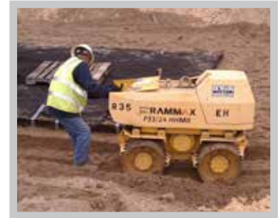
Fig. 17 Vibratory compaction of side backfill is ALWAYS REQUIRED, regardless of what backfill material is used.
