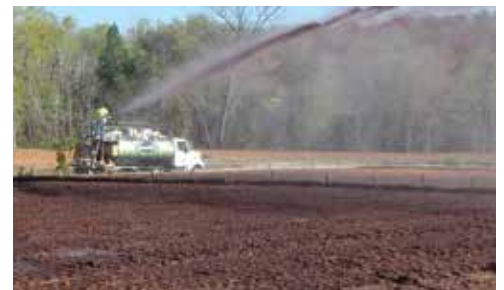
Hydraulically applying ProGanics is more cost-effective than typical topsoil or compost applications, and it overcomes soil deficiencies better than alternative Biotic Soil Amendments.
