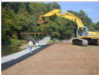
This is the more traditional method of installation. In the case of this project, it just wasn't feasible.
