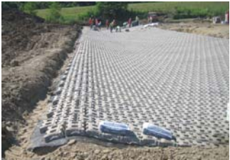
All block placed and laced. The place and lace method make for a very nice looking installation.
