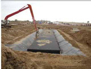
The Atlantis D-Raintanks were then wrapped in fabric and a sand biofiltration layer was placed.
