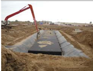
The Atlantis D-Raintanks were then wrapped in fabric and a sand biofiltration layer was placed.
