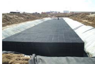
1,079 Triples Atlantis D-Raintanks were assembled and placed on the a 6" sand layer on liner bottom.
