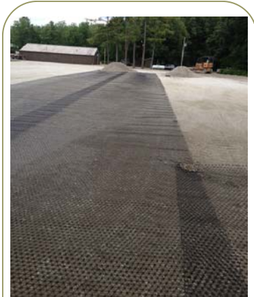
Triax Geogird was placed on top of the soft subsoil and greatly shortened the construction time.
