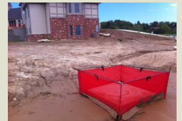
Over 3 acres of disturbed land drain into this area inlet. Note the sediment build up.
