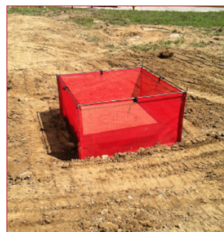
"Big Red" AI Protector, recently installed with trenched in bottom and tight sides.
