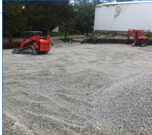
4 Clean rock is used for backfill over the tanks. This rock will be used for filtering the water and provides additional storage.
