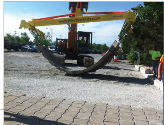
6 An excavator uses PaveDrain's spreader bar to easily lift and place large sections of block onto a compacted rock base.
