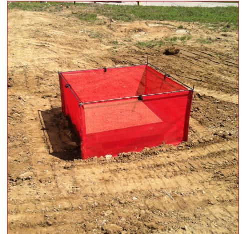
"Big Red" AI Protector, recently installed with trenched in bottom and tight sides.
