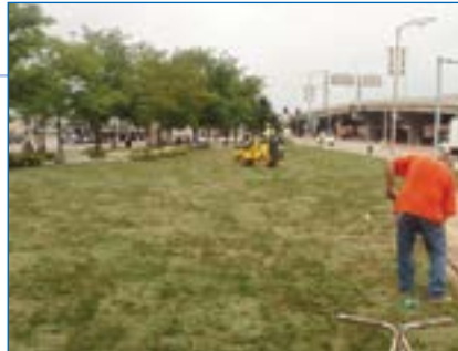
4 Sod was placed on top of the soil filled cells and rolled.
