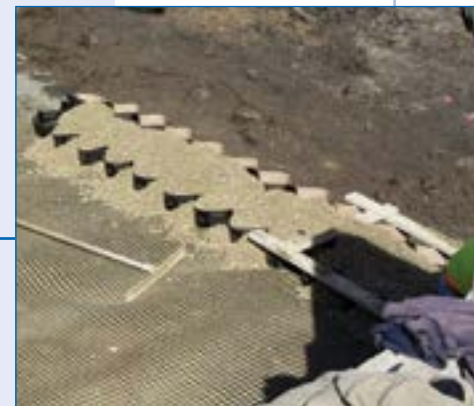
2 Geogrid layers utilized for reinforcement. The wood stretcher frame is used to hold the Geoweb open as material is infilled.
