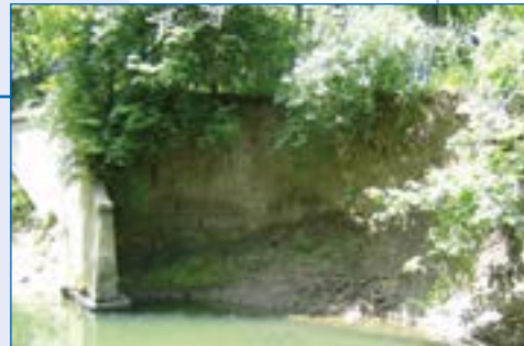
1 Pre construction photo showing the abutment erosion and the loss of the trail.
