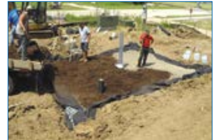
5 Mulch is being installed while hydraulic conductivity test is being performed to insure flow rates.
