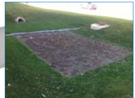
7 After sodding, the system was opened up, tested again for flow, and "commissioned" for use.
