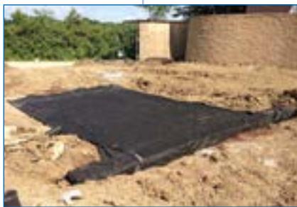
6 Since ground around Focal Point is not stabilized, the system is completely sealed off to keep sediment from plugging system.
