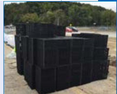
1 ACF R-Tanks for underdrain.
