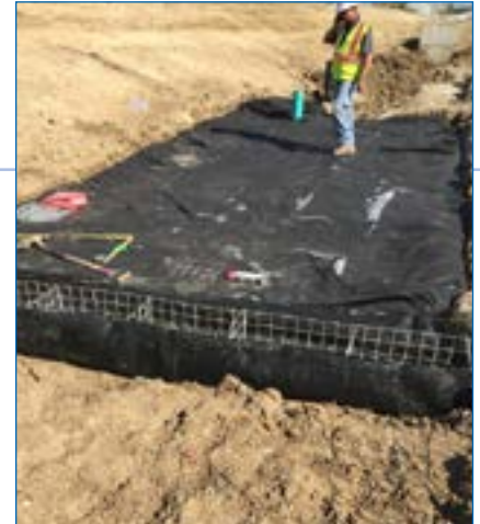
5 Gabion Level Spreader.
