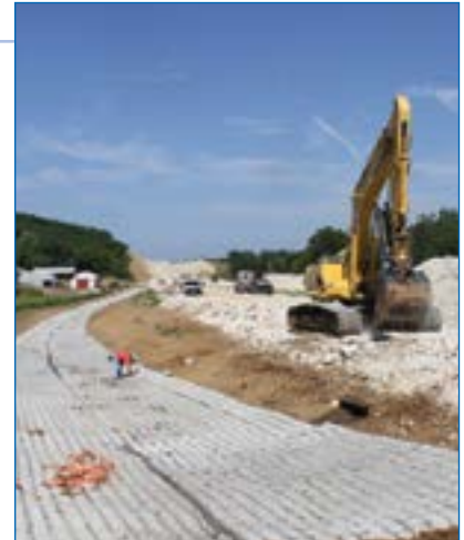
5 Upstream toe of the Flexamat buried in an anchor trench to prevent undercutting.
