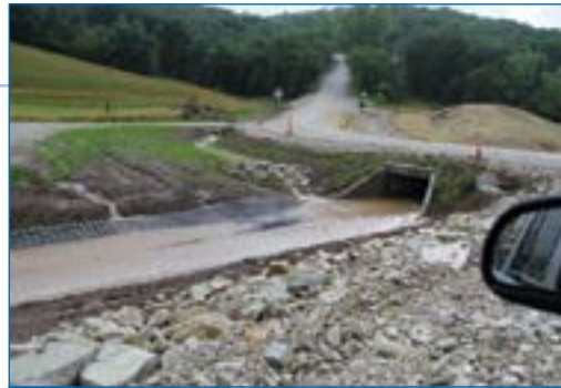
4 Sudden downpour with only 1/2 of the channel protected.
