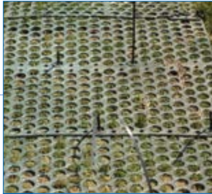
4 ScourStop can be cut around irregular shapes, such as this lamp-pole base.
