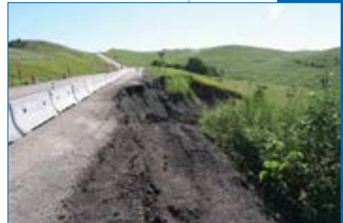
1 Photo Verdigre east slide pre repair.
