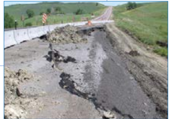
6 Saturated soils cause slope failure.
