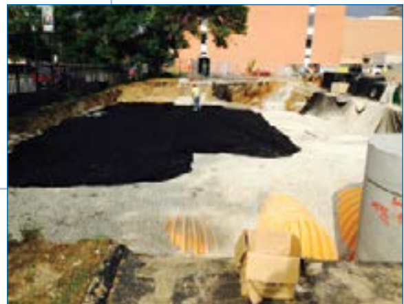
7 Excavation for BMP is backfilled completely with clean aggregate and protected with non-woven geotextile.
