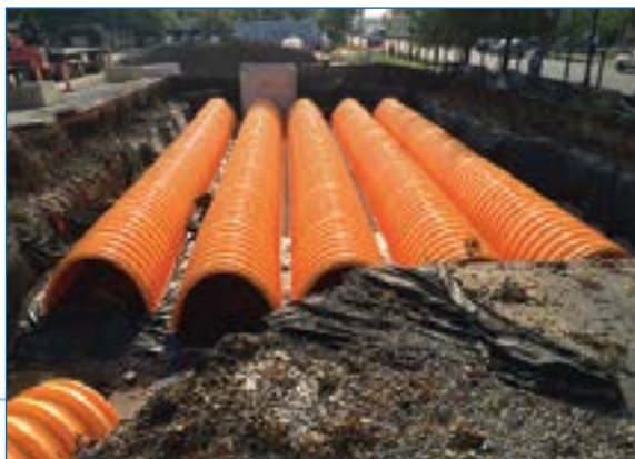
6 Arch chamber installation is completed. Notice woven geotextile placement to avoid scouring of clean rock.
