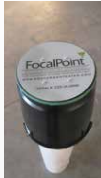
Figure 14: Cut inspection port to appropriate height stated on plans. Seal the opening on top of the pipe with the FocalPoint Inspection Port Cap or temporary lid
