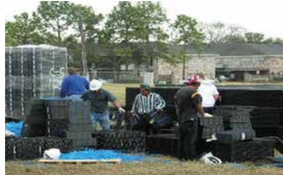
Figure 3: Assembling on site during excavation will increase speed once the excavation is completed
