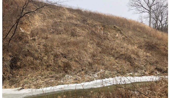
Image of the project site before intervention showing the slip surface of the slope within the pipeline ROW.
